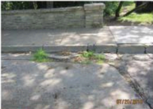
Example of damage to bridge infrastructure
