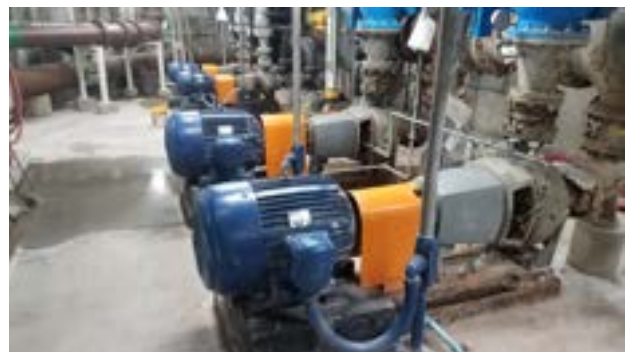
Pump motors in blue at one of the plant buildings
