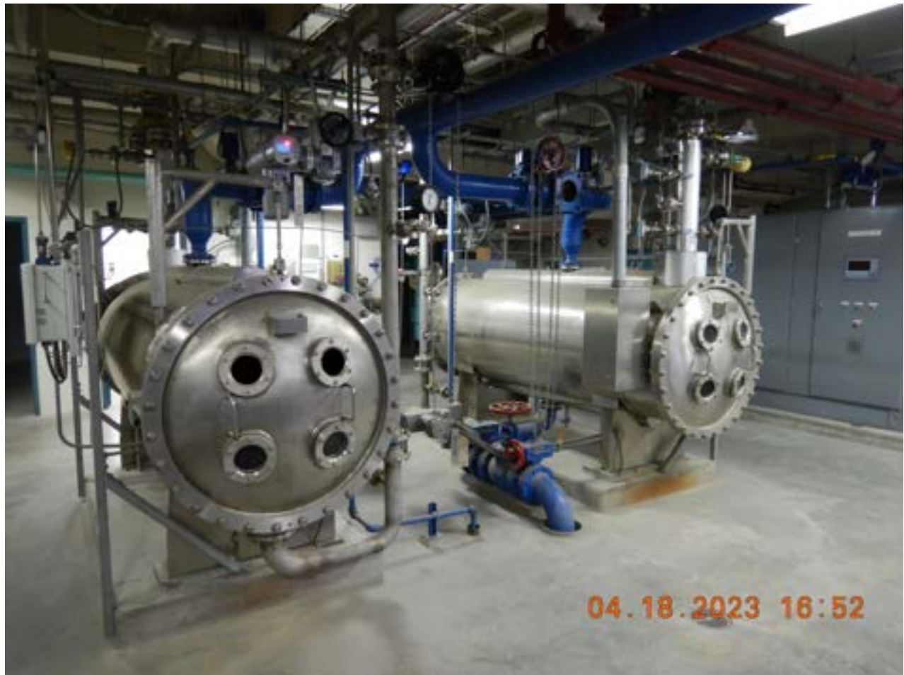
Figure 1: City of Fargo ozone generators
