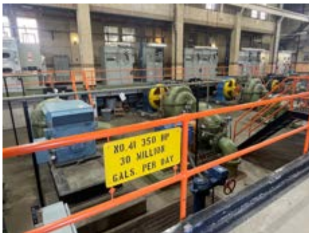
Pumps and pump starting equipment at pump station no. 5
