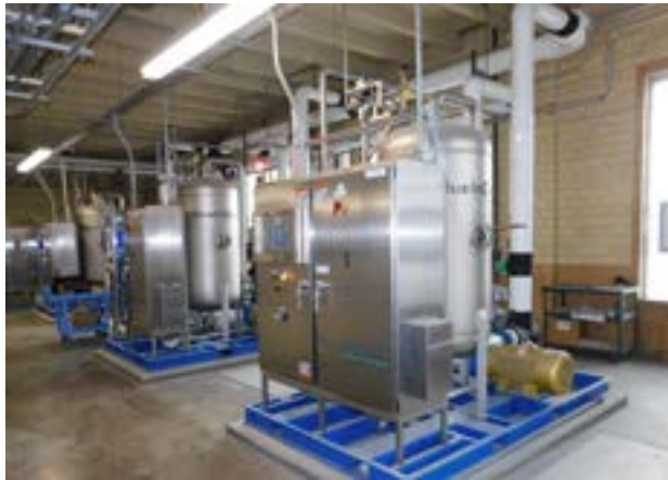
Recently installed CO2 equipment
