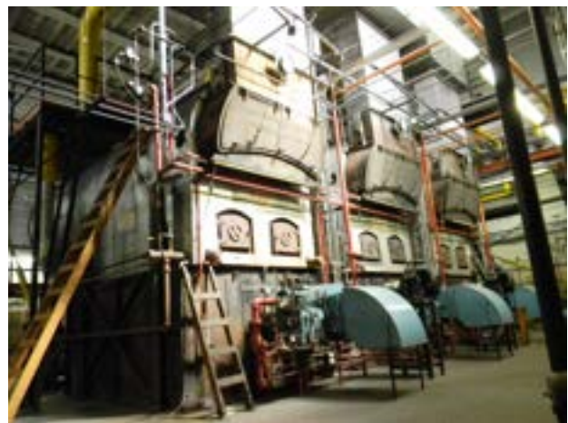
Heating boilers at pump station no. 6
