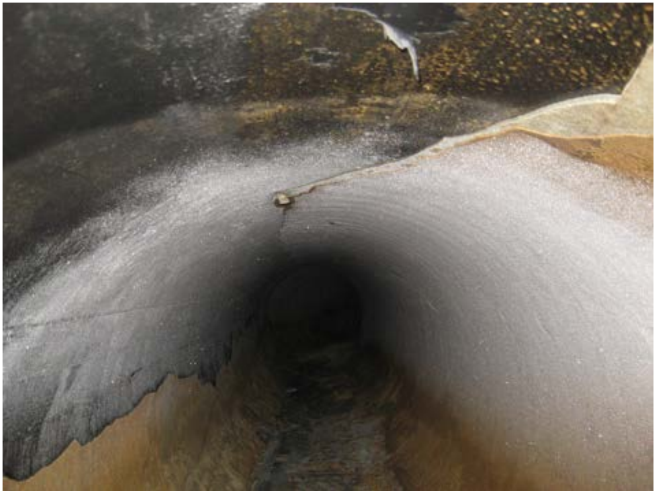
Franklin Avenue bridge main interior showing the lining material failure.
