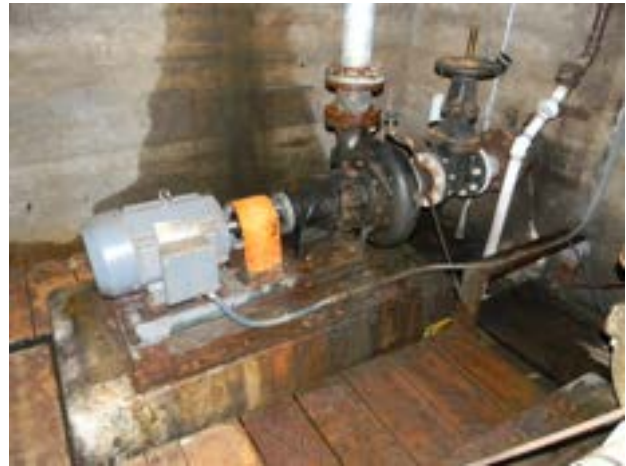
Sanitary lift station at
