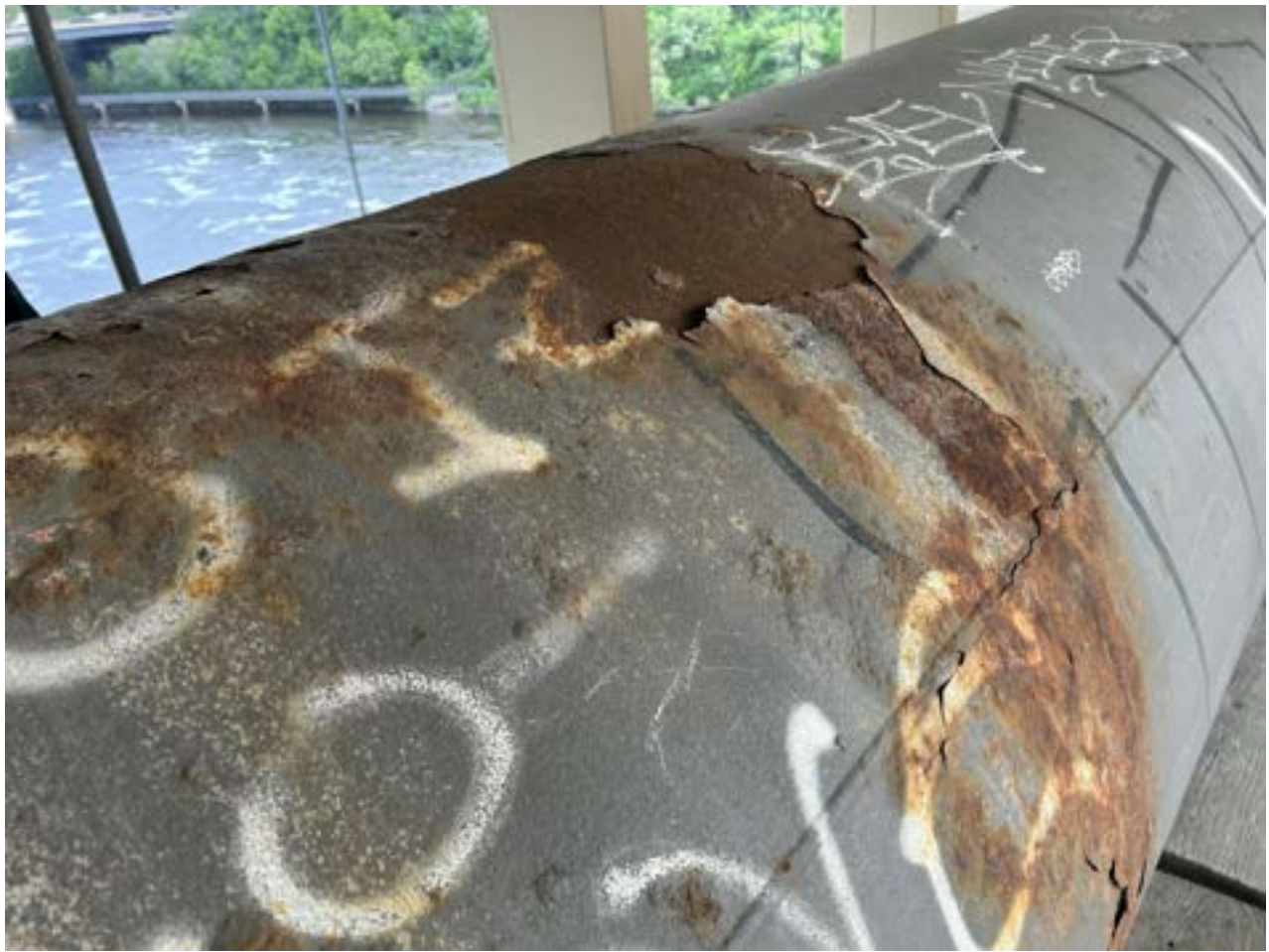
Franklin Avenue bridge main over the Mississippi River showing typical corrosion from road salt from the bridge deck above
