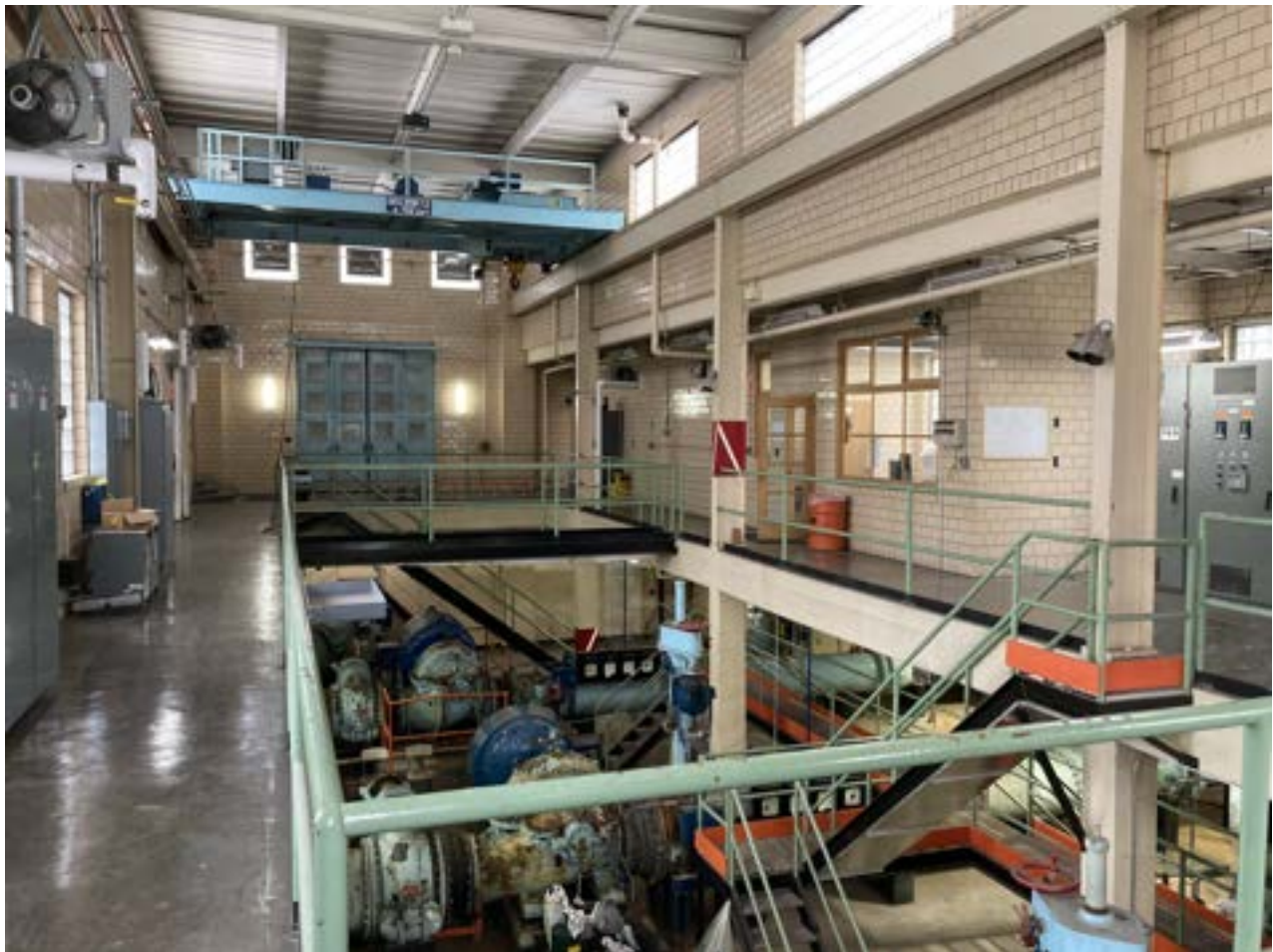
Pump station No 7 where the current NE high service pumps are located.
