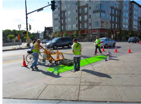
Figure 16-8: A contractor installing preformed thermoplastic on 15 th Avenue Southeast at 4 th Street Southeast
