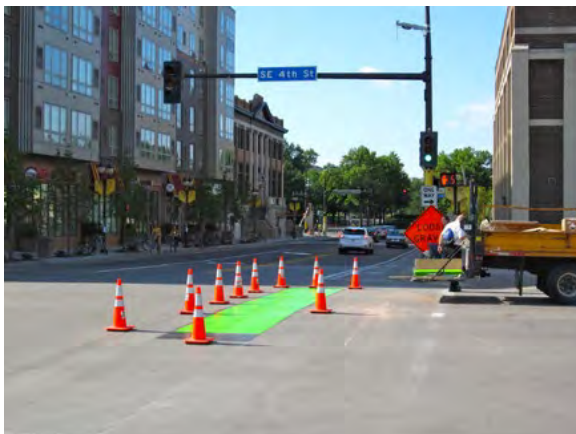
Figure 16-9: Preformed thermoplastic material shortly after installation on 15 th Avenue Southeast at 4 th Street Southeast
