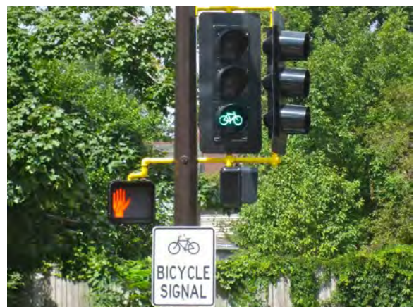
Figure 8-9: 12-inch signal heads and “Bicycle Signal” signing on northbound 5 th Street Northeast approach at Broadway Street Northeast after installation
