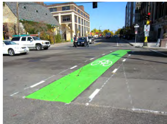
Figure 16-10: Preformed thermoplastic material shortly after installation on 15 th Avenue Southeast at University Avenue Southeast
