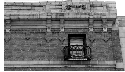
A terra cotta parapet, cornice, and paired brackets crown the Fawkes Auto Company (1912) at 1633-37 Hennepin Avenue.
