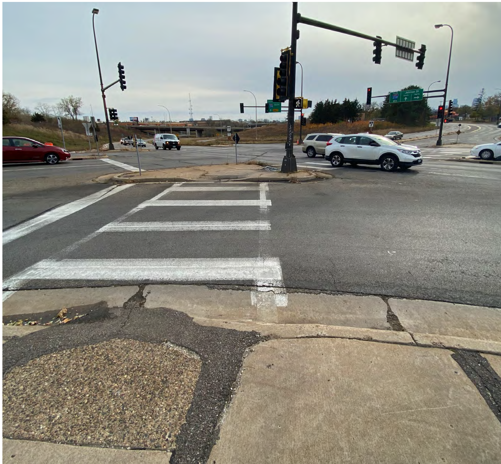
Patchy sidewalk does not meet current ADA standards
