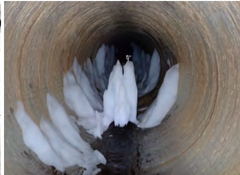
Ice buildup in tunnel
