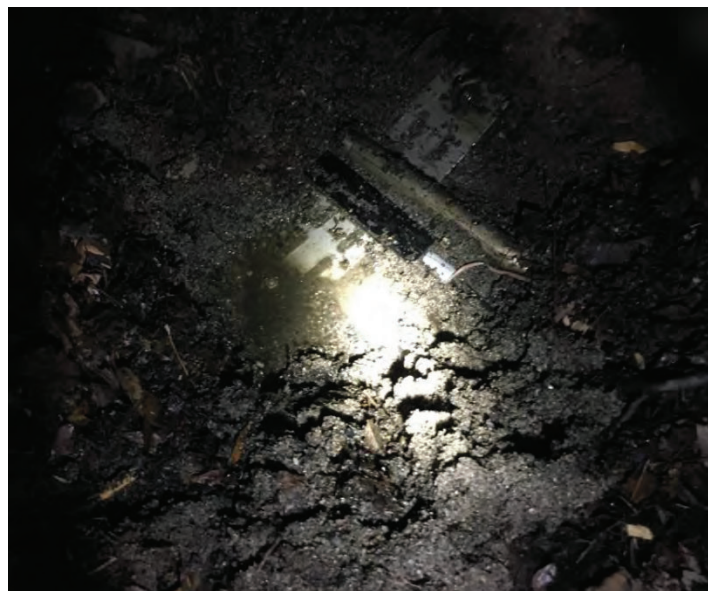
Figure 25-4. A 2019 photograph of the upstream Powderhorn Inlet South offset AV probe and intake strainer after removing 8” of sand and debris.
