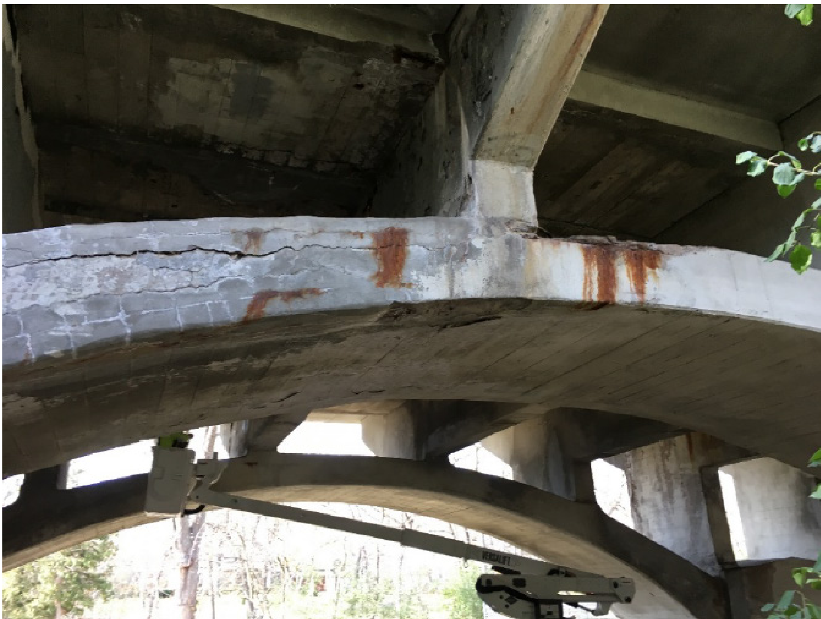
Major Crack and Concrete Deterioration on Arch Rib
