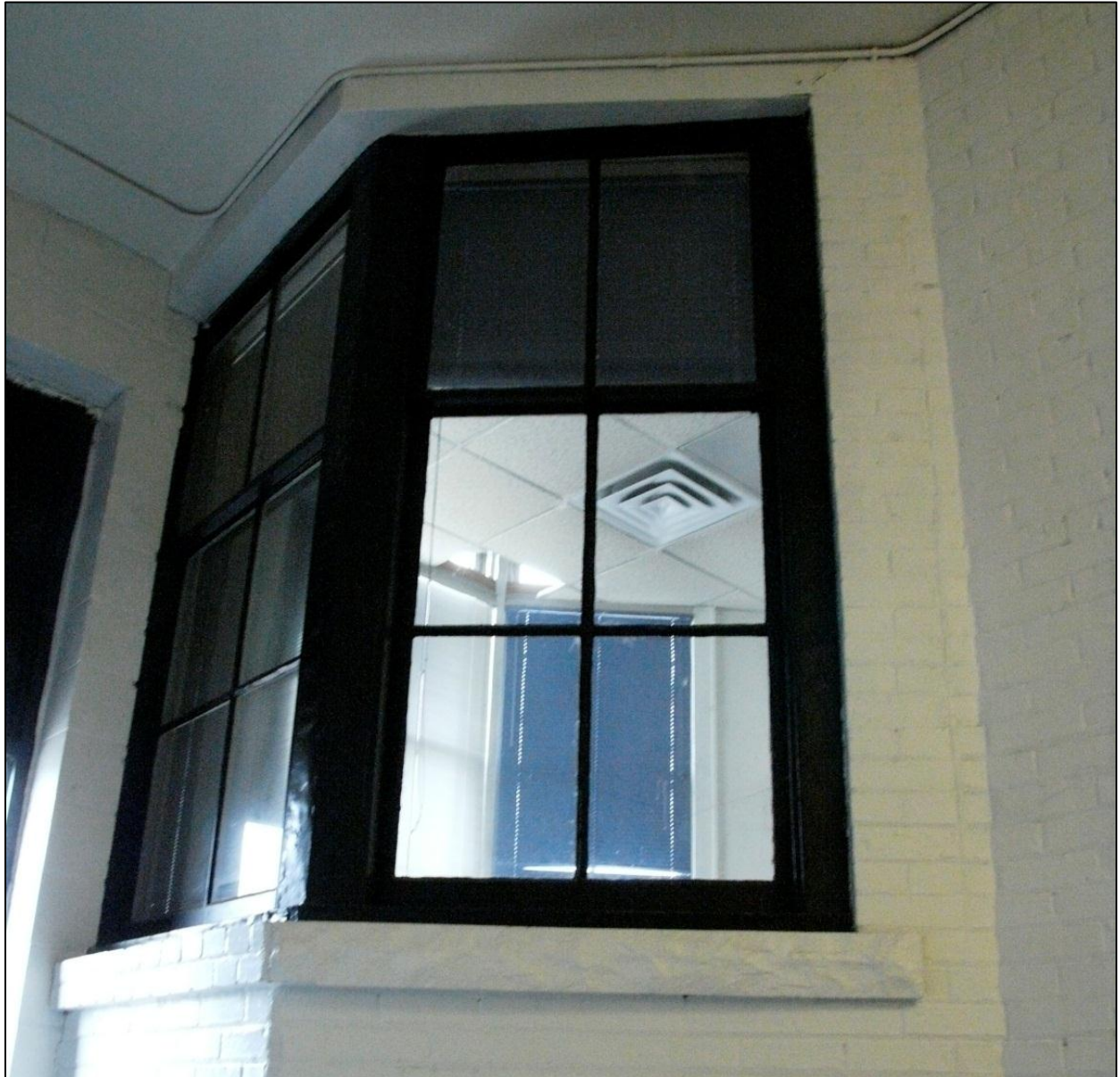
Figure 7. Interior portion of the five-part bay window enveloped by the addition into the present main entry. Source: CPED files
