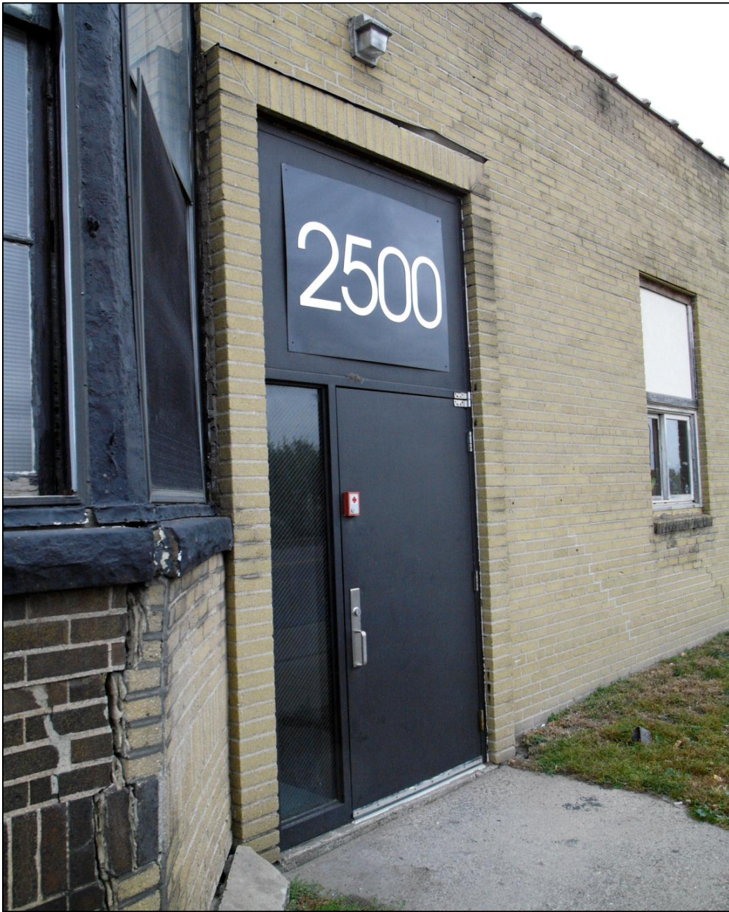
Figure 5. Main entry off of Washington Avenue. Note the use of tan brick in the bay window; the addition envelops the south exterior wall of the 1914 building. Source: CPED files.
