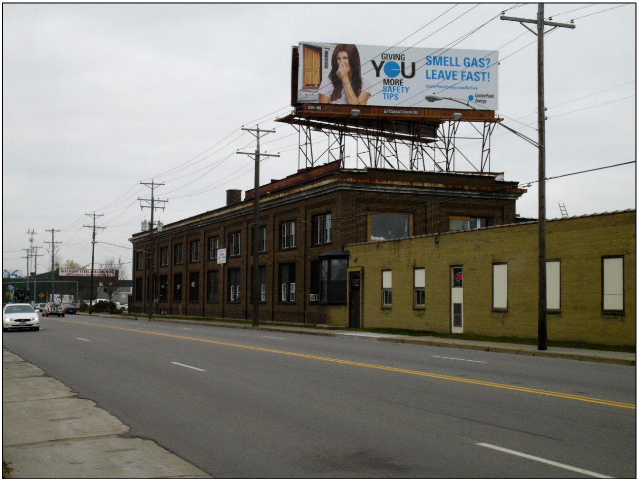
Figure 1. North Side Station, Washington Avenue North frontage, view from the southwest. Note the billboard on top of the 1914 building, the deteriorated cornice, the 1954 addition in light tan brick adjacent to the protruding bay window. Note also the replacement windows and wood panel infill. Source: CPED files.
