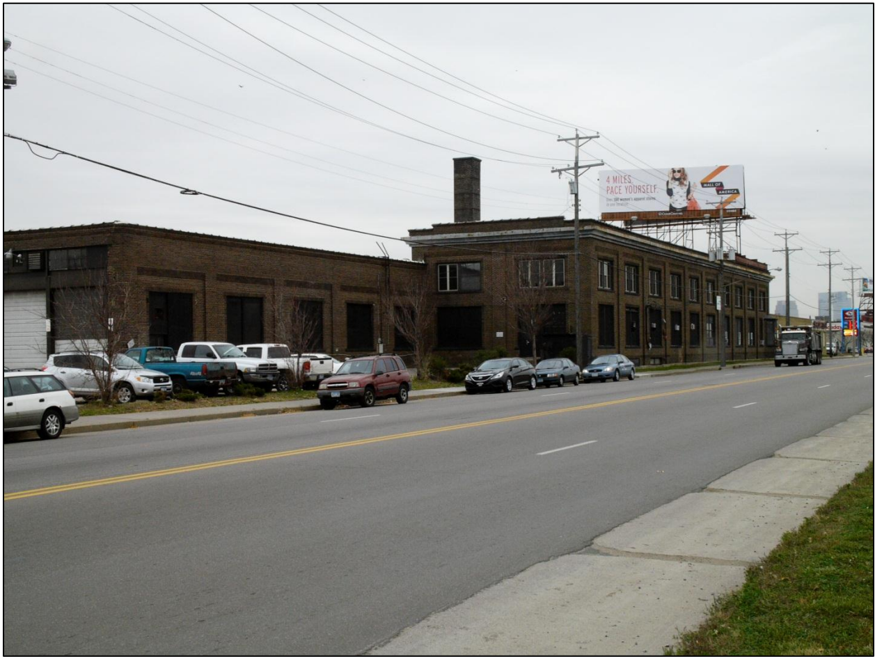
Figure 2. North Side Station, Washington Avenue frontage, view from the northwest. Note the chimney, the parapet, the metal cornice, the wood infill panels and replacement windows and shed bay doors. Source: CPED files.
