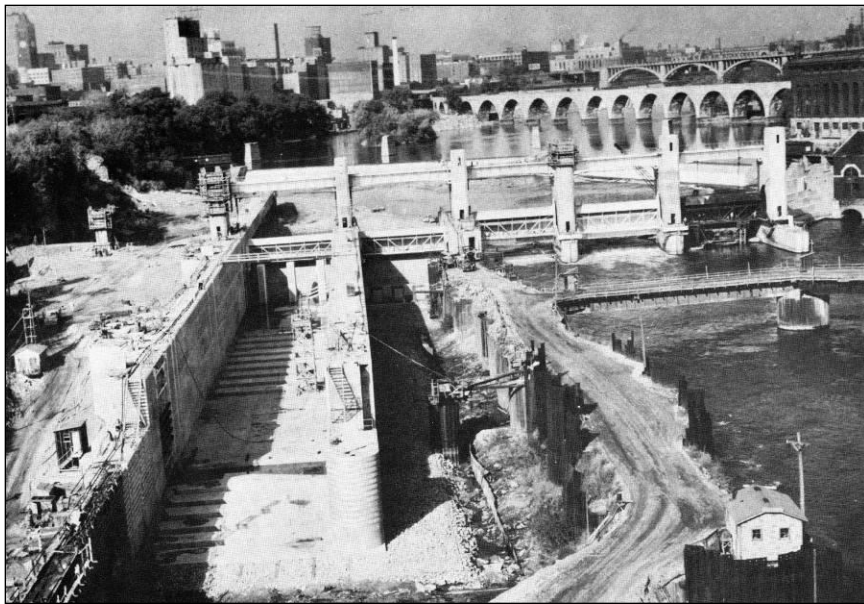
Lower Saint Anthony Falls Lock and Dam under construction, ca. 1955. (Upper Harbor: Minneapolis and the Future. . . .)
