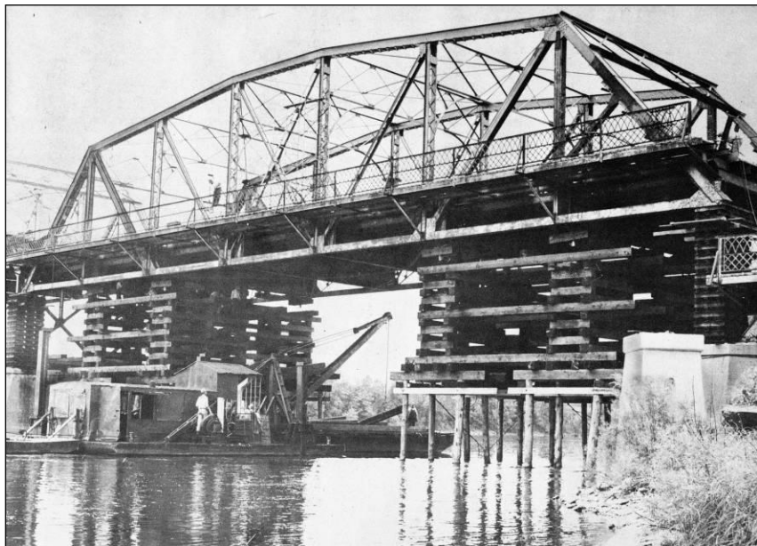
Raising one span of the Plymouth Avenue Bridge to accommodate barge traffic in the Upper Harbor, ca. 1955. ( Upper Harbor: Minneapolis and the Future. . . . )
