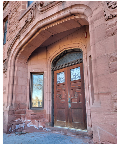
The historic wood door is present at 2116 2nd Ave S. It has a decorative frame and a leaded transom window above. It is important to preserve these features.
