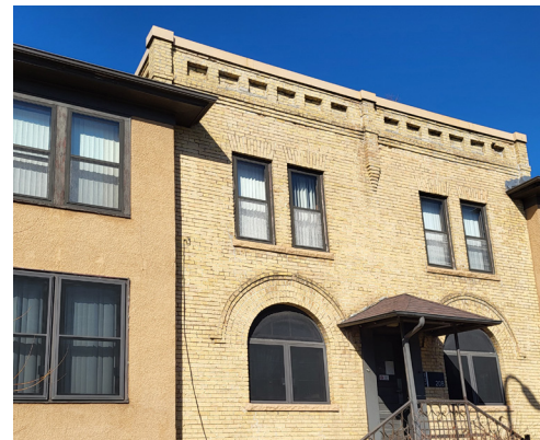
The storm windows at 206, 208, and 210 26th St E are pre-finished metal. Storm windows help retain heat inside the building.
