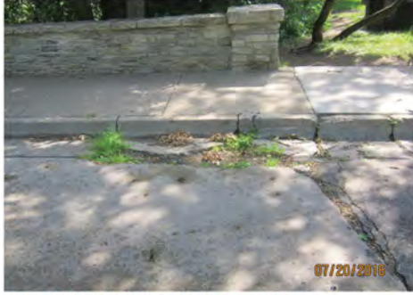
Example of damage to bridge infrastructure
