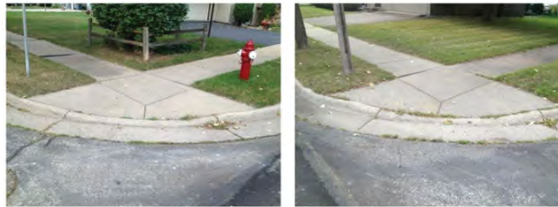
Some pedestrian ramps do not meet current ADA standards for accessibility.
